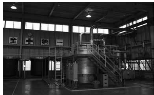
Fig.2. Akita office (liquefaction plant)
